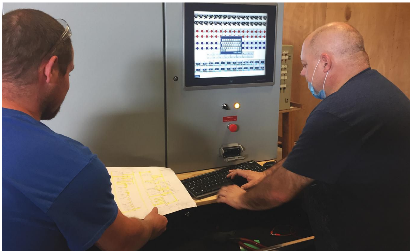
FIGURE 2. Technicians perform a full FAT for a system consisting of a burner management/combustion control system, fuel skid and selective catalytic reduction (SCR) system.
