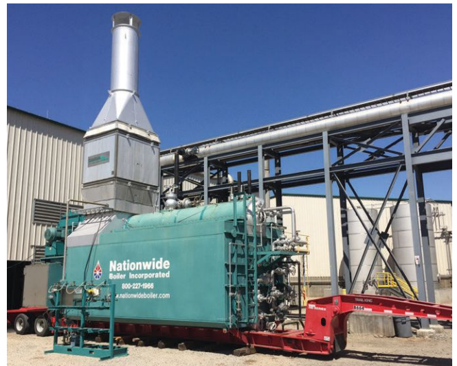
A 77,000 lb./hr. trailer-mounted saturated steam rental boiler installed with an anhydrous ammonia SCR system – no structure required.
