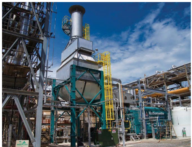
This 110,000 lb./hr. trailer-mounted superheated steam boiler is recognized as one of the world's largest. It is installed with a urea-based SCR system, economizer, and support structure.
