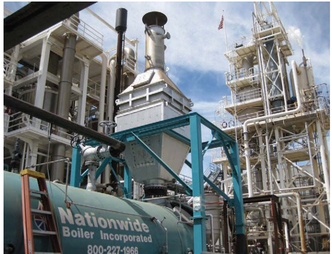
A firetube boiler with an SCR system rental.
