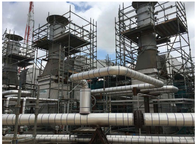
Multiple ground-mounted rental SCR systems installed on 75,000 lb./hr. superheated steam rental boilers.
