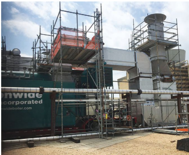
A 75,000 lb./hr. superheated steam rental boiler installed with a ground-mounted, urea-based SCR system.
