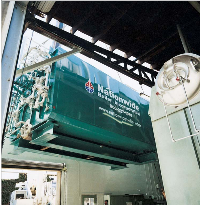
50,000 lb/hr package boiler with ultra low NOx burner being lowered into the boiler room.
