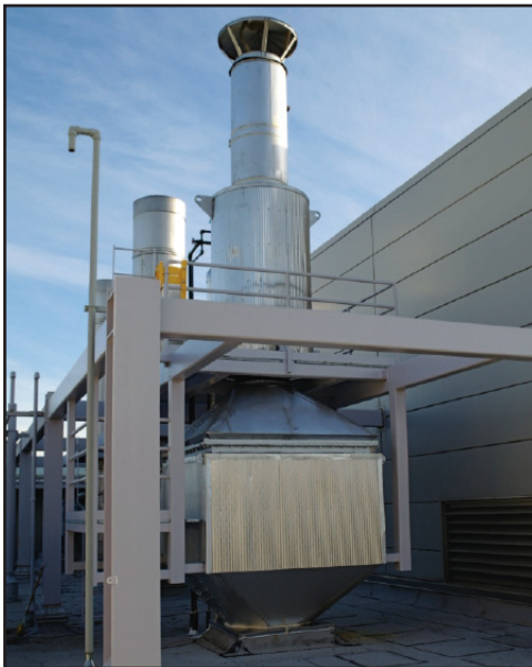
1,000 HP boiler with a CataStak™ SCR system. The unit tested at 1 ppm NOx and achieved full capacity with an improved operational efficiency.
