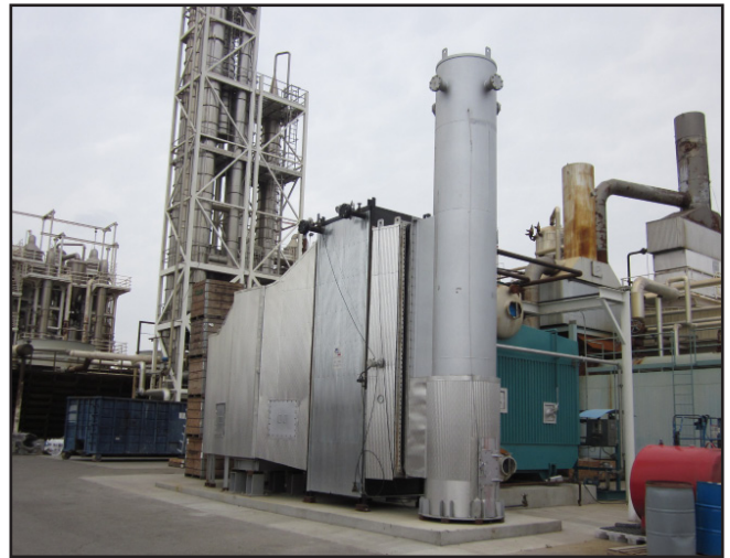
82,500 lb/hr BPS boiler rental.
