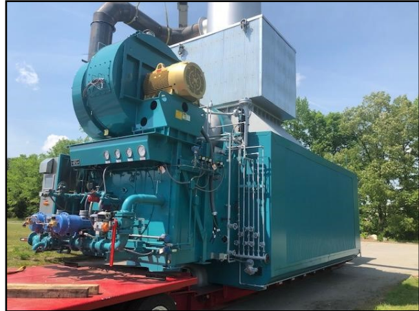
This boiler can be de-rated for improved emissions performance!
