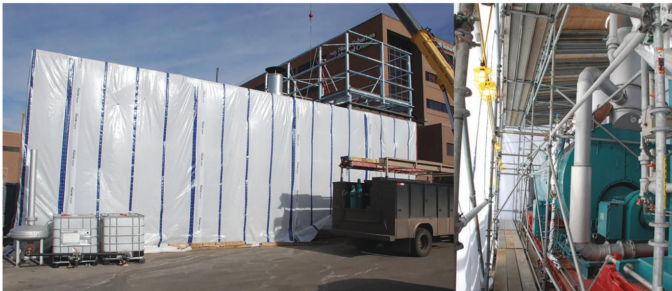
A temporary enclosure protects this mobile steam plant, which contains a boiler, feedwater system, water softener, chemical-feed system and control panel.
