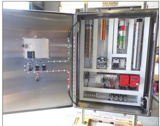
A PLC-based burner management system and parallel positioning combustion control panel (internal view).
