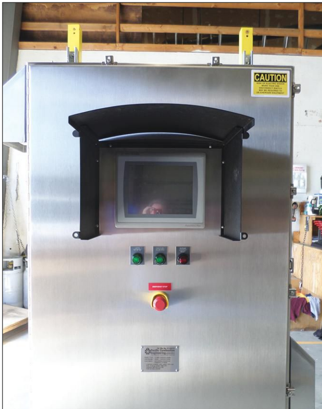
A PLC-based burner management system and parallel positioning combustion control panel with a touch-screen operator interface.
