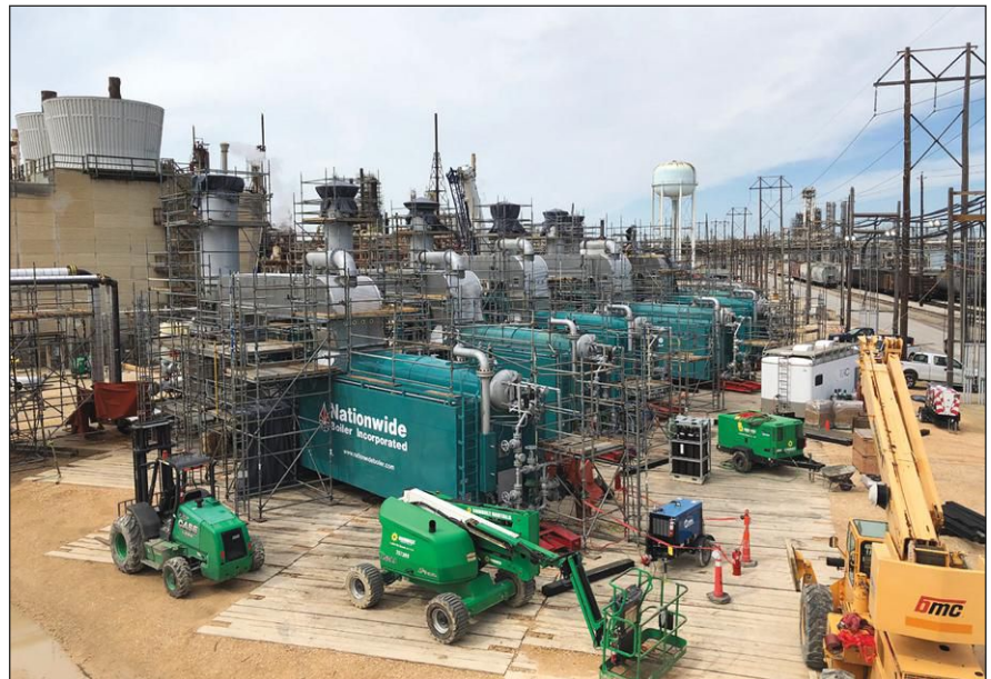
Figure 1: With multiple obstacles to overcome, Nationwide Boiler designed a solution to meet the customer's operating parameters, installation restrictions, and swift operational timeline.
