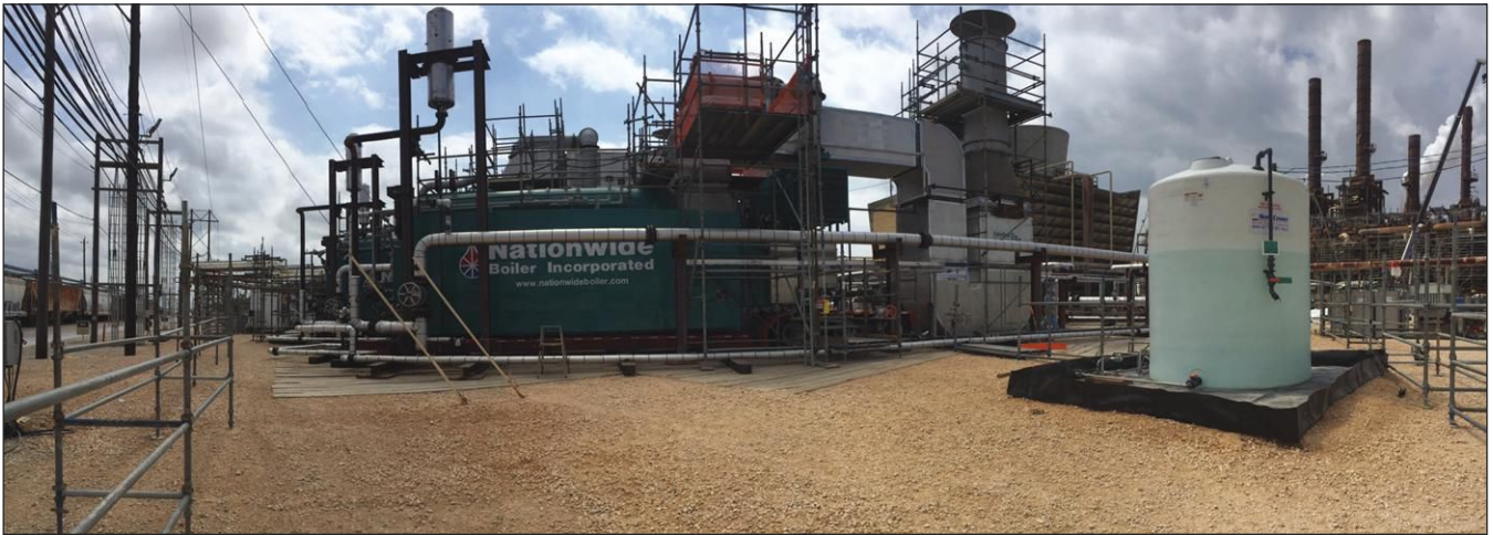
Figure 2: With inventory and availability both a major factor in the delivery and timing of this project, Nationwide Boiler was able to reserve and prepare six 75,000 lbs./hr., 750 psig/750°F superheat, trailer-mounted, package, watertube, rental boilers to make up the total steam demand.
