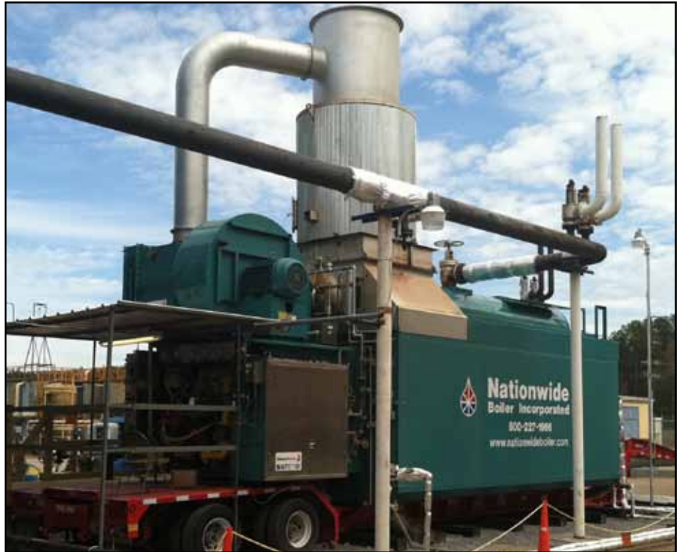
82,500 lb/hr trailer-mounted boiler rental at Columbus, MS.
