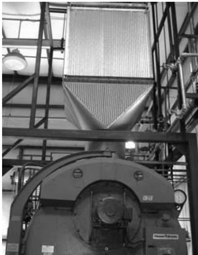
Retrofit of a 700 hp natural gas-fired Cleaver-Brooks firetube boiler with a CataStak SCR System. The unit was tested at less than 0.5 ppm NOx.
