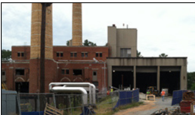
Top: 82,500 lb/hr trailer-mounted rental boiler adorned with Duke University's Blue Devil logo.
